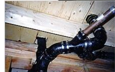
Cast-iron drain, waste and vent piping
